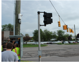
Traffic lights and controller in Ann Arbor, Michigan
