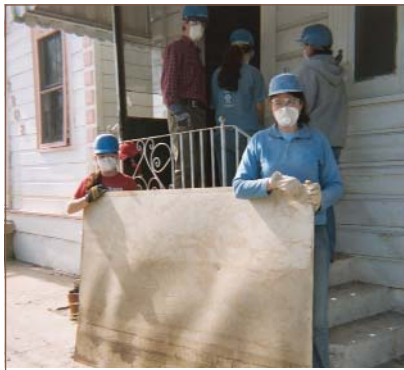
These Circle K members spent part of their winter break in New Orleans, gutting homes damaged by Hurricane Katrina in 2005.
