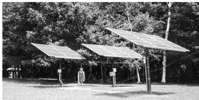
Professor Delano's family has two kinds of renewable energy systems at their home, including the solar panels shown in this image that generate about 35% of their electricity. During occasional power outages due to storms, the family's comfort is maintained (e.g., following the electrical outage in December 2008 due to the ice storm that knocked out electricity for nearly 7 days). Students in his UFSP 100 course have visited his home to see these renewable systems in operation.
